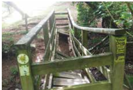
Footbridge in south-west Herefordshire, closed since August 2020 by a TTRO because the council has failed to mend it. Photo: David Howerski.
